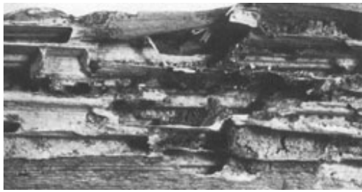
Termite damage in timber
